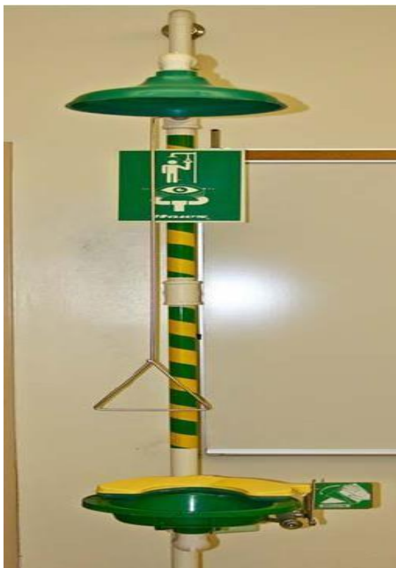
Figure 1: Safety shower/eye wash combination located in the front of classroom.
